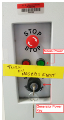
Figure 6. D4 Front control panel.
