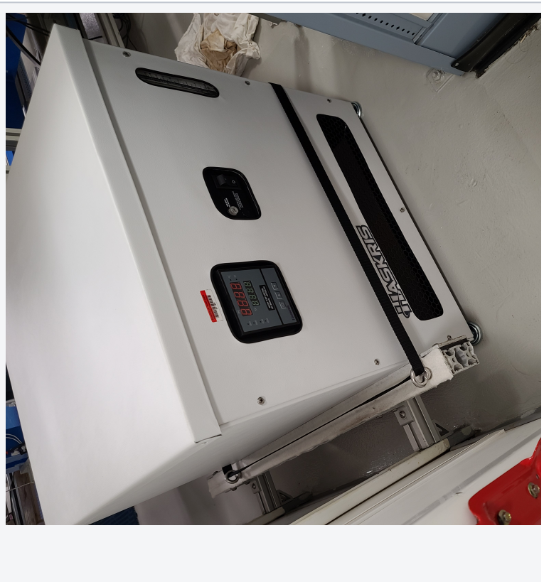
Figure 1b: Main Haskris Water Chiller (water cooled). This unit is located at the forward end of the paleomagnetism lab and requires ship chill-water.
