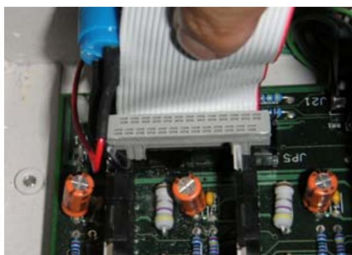
Figure 4. Serial Cable Connector to the Main Control Unit.
