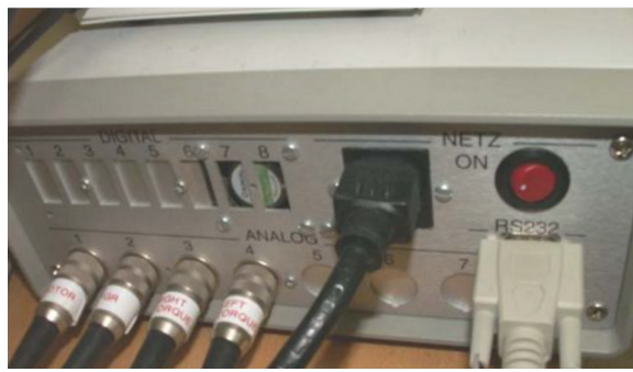
Figure 5. Back View of FL2SS Controller.
