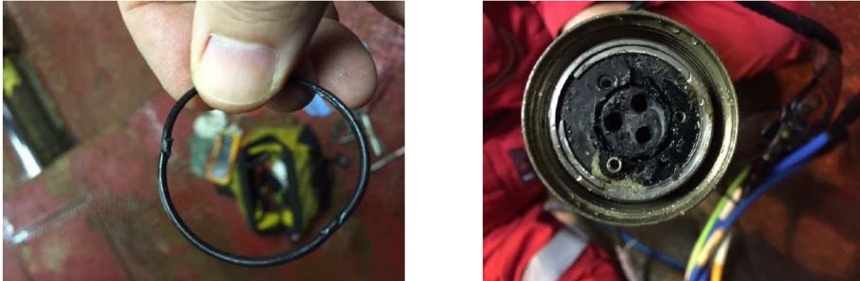
Figure 9. Damage to O-ring and Connector due to Failed O-ring.
