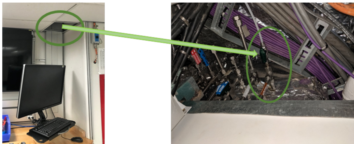
Figure 5. Ceiling panel with He shut-off valve.
