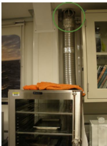
Figure 9. Exhaust tubing and the butterfly valve control (circled in green). The desiccator boxes are to the left of the exhaust tubing.
