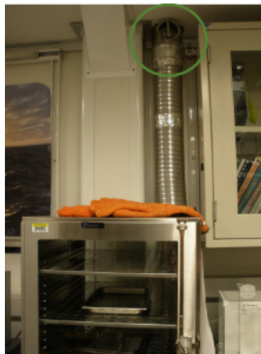
Figure 40. Exhaust tubing and the butterfly valve control (circled in green). The desiccator boxes are to the left of the exhaust tubing.
