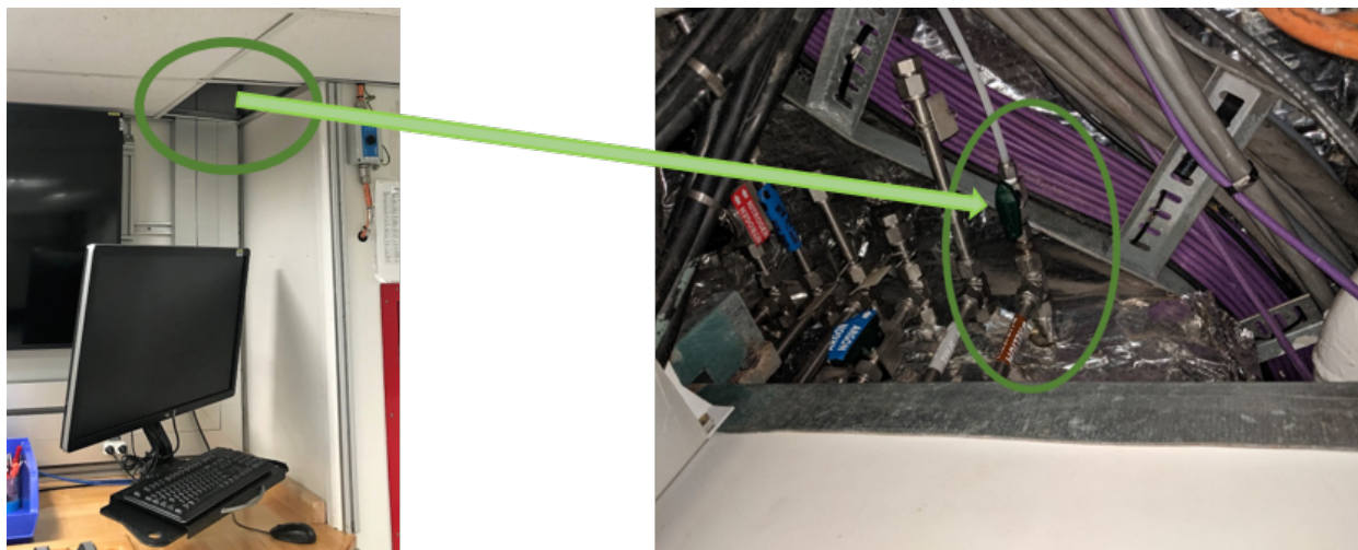
Figure 5. Ceiling panel with He shut-off valve.
