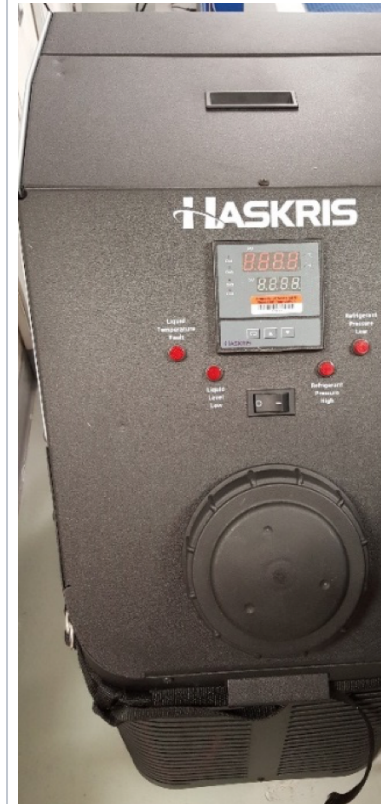
Figure 1b: Backup Haskris Water Chiller (air cooled). This unit is located at the forward Core lab under the Forward Description in the unit is air cooled, it will generate heat space
