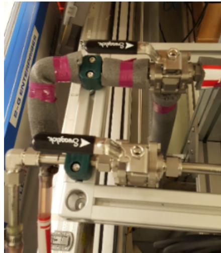
Figure 10: Valve positions when using ship's chill water for cooling the SRM compressor.
