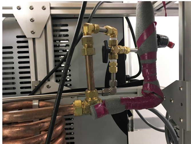
Fig 2b: A bypass valve for the tube-in-tube heat exchanger coil was installed on Exp. 379T (July 2019). This valve allows you to cut the heat exchanger out of the cooling loop and run directly on ship's chill water entirely. Opening or closing this valve gives you approximately 10F of oil temperature change. The pictured valve position indicates the heat exchanger is included in the cooling loop.
