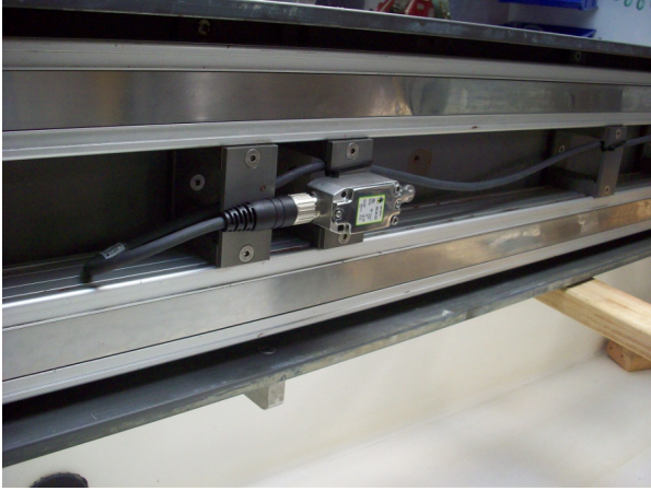
Left: Travelling block limit switch, one of two. Right:
