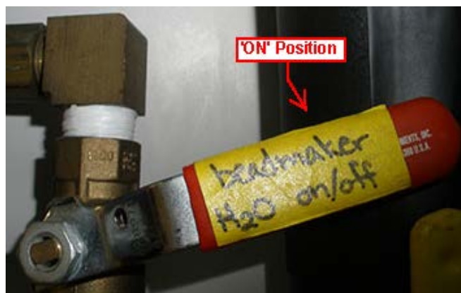
Figure 48. Water in on position.
