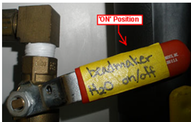
Figure 32. Water in on position.
