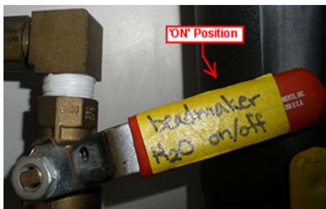
Figure 47. Water in on position.
