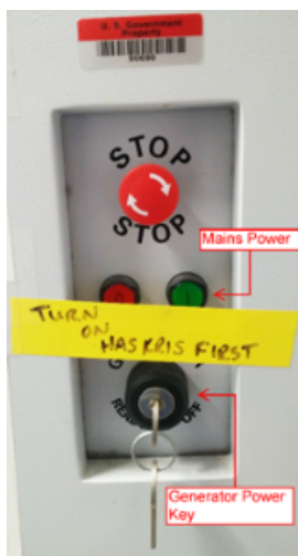
Figure 4. D4 Front control panel.
