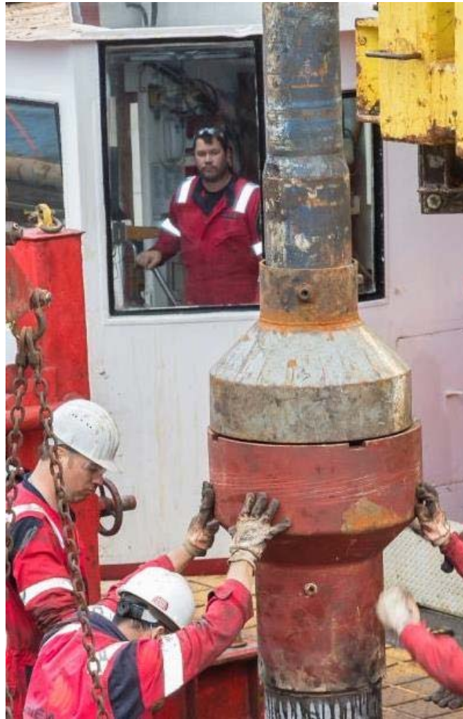
The Platform and Funnel Guide (gray) on top of the Mock Hanger (red).
