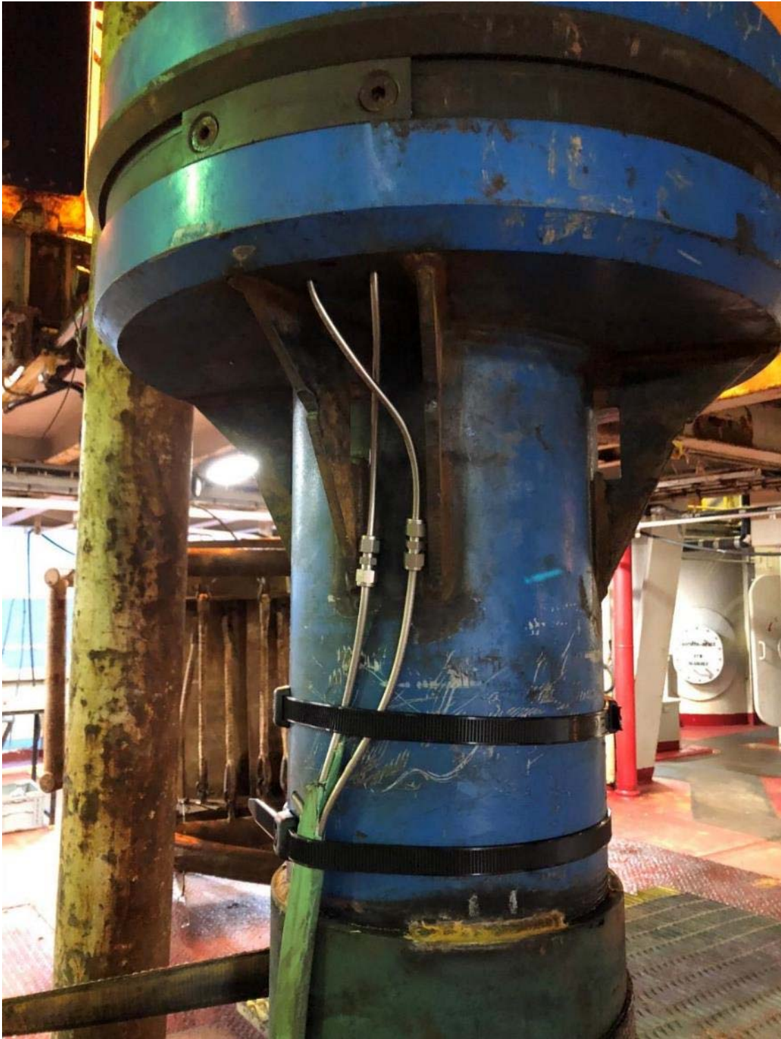
The plumbing on the U1519B ACORK. The umbilical was brought around to the pass-throughs on the Base Adapter to make the connections simpler and quicker.
