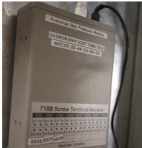
Data acquisition device labeling
