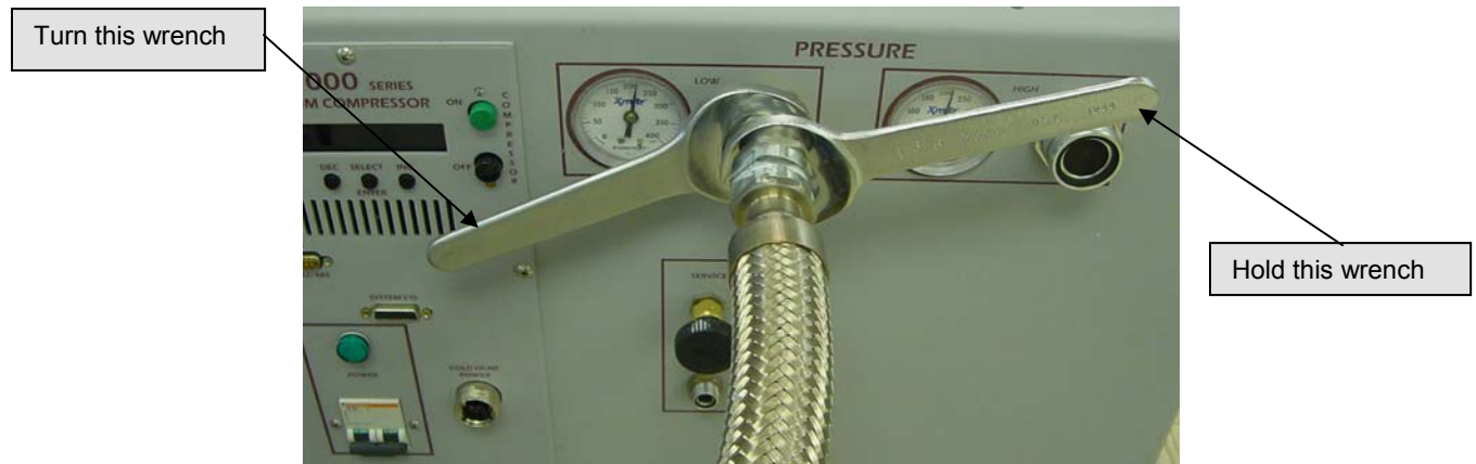
Figure 7-1: Disconnecting flex lines from a compressor package
