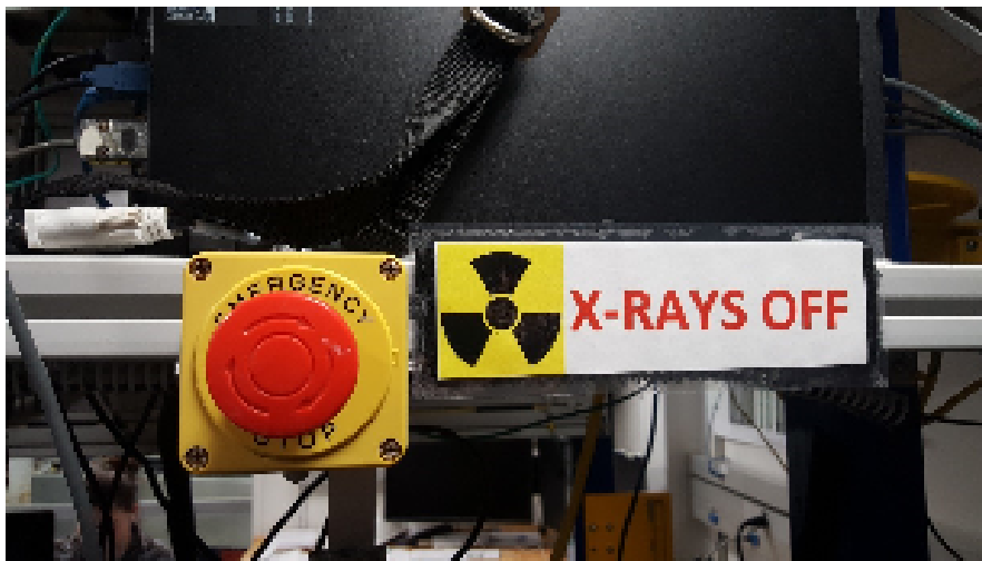
Figure 7-X-ray logger Emergency Shut Off Switch.
