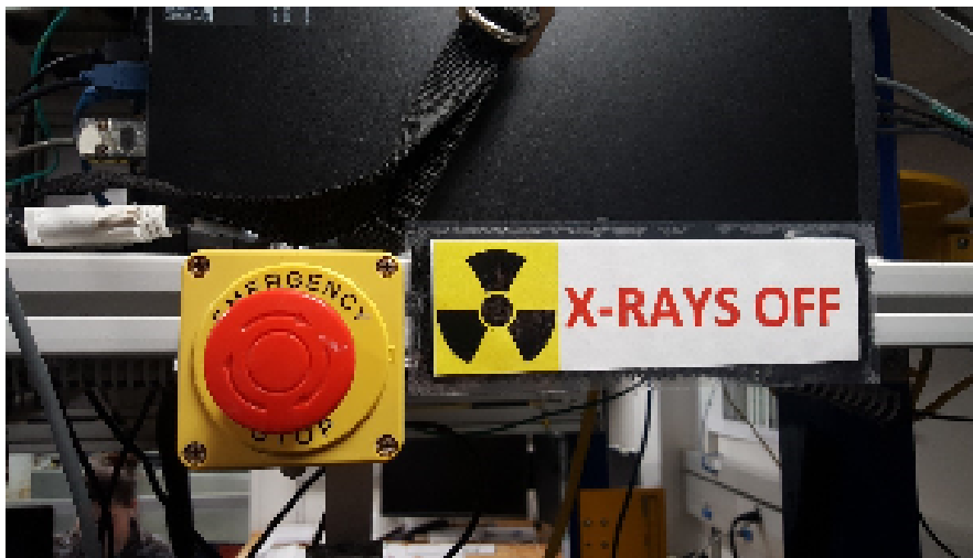
Figure 7-X-ray logger Emergency Shut Off Switch.
