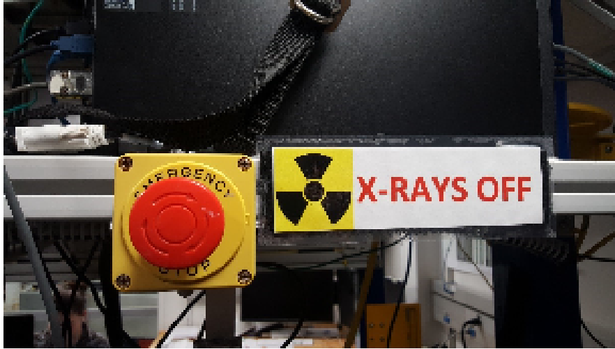
Figure 50. X-ray logger Emergency Shut Off Switch.
