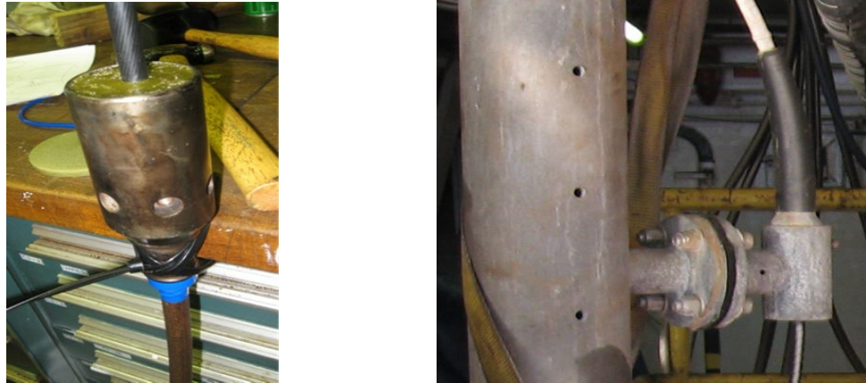
Figure 6. Cablehead Preparation and Mounting.
